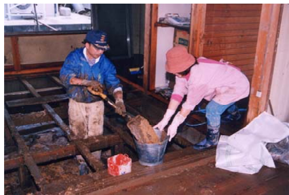
Residents remove silt from their homes
