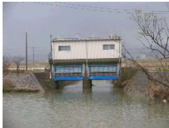
Maruyama River's sluice pump system
